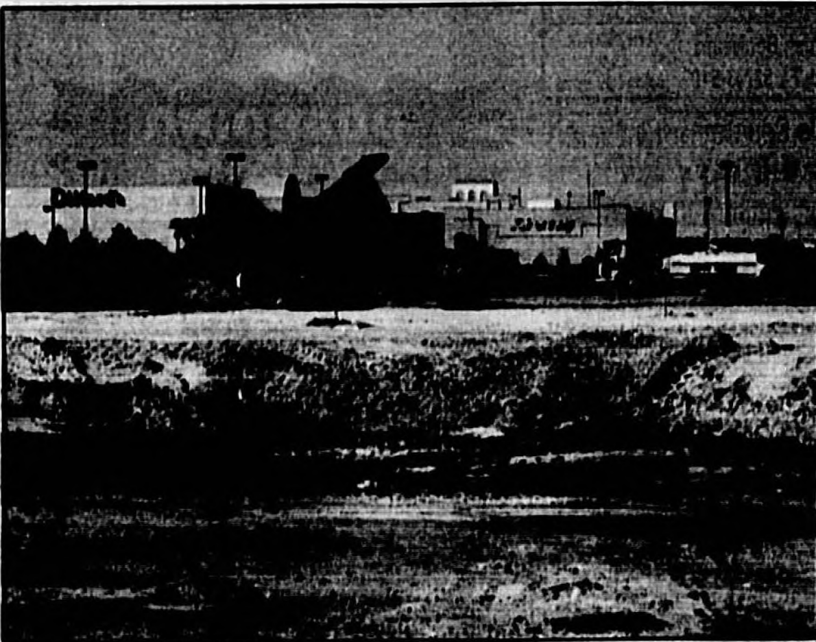
Construction has begun on the new Towne Center Plaza off Interstate-4 on Towne Center Boulevard.
