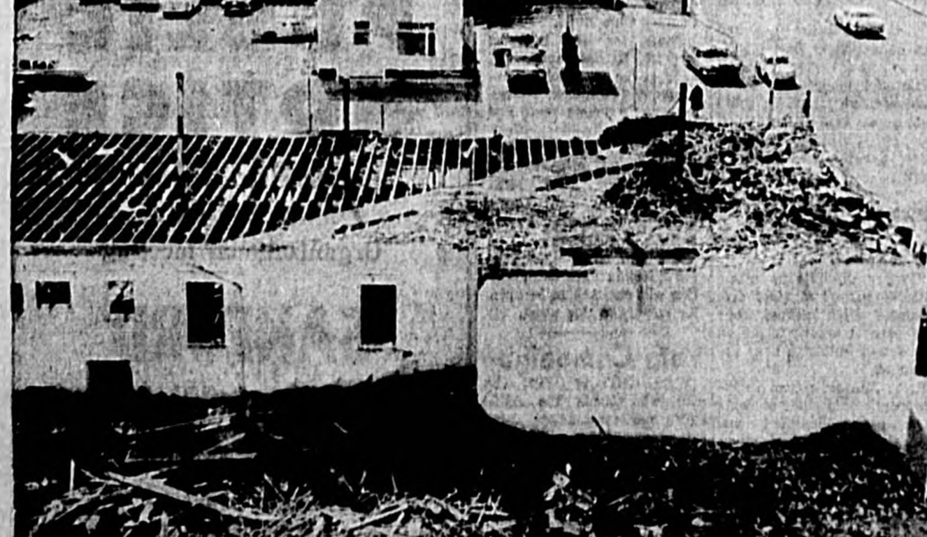
THE OLD FLORIDA HOTEL at Park Avenue and Second Street is almost "no more," as shown in this photo from the fifth floor of the Sanford Atlantic National Bank building. The hotel is being razed to make way for a bank parking lot and, in the future, a new bank addition. (Miami Photo)
