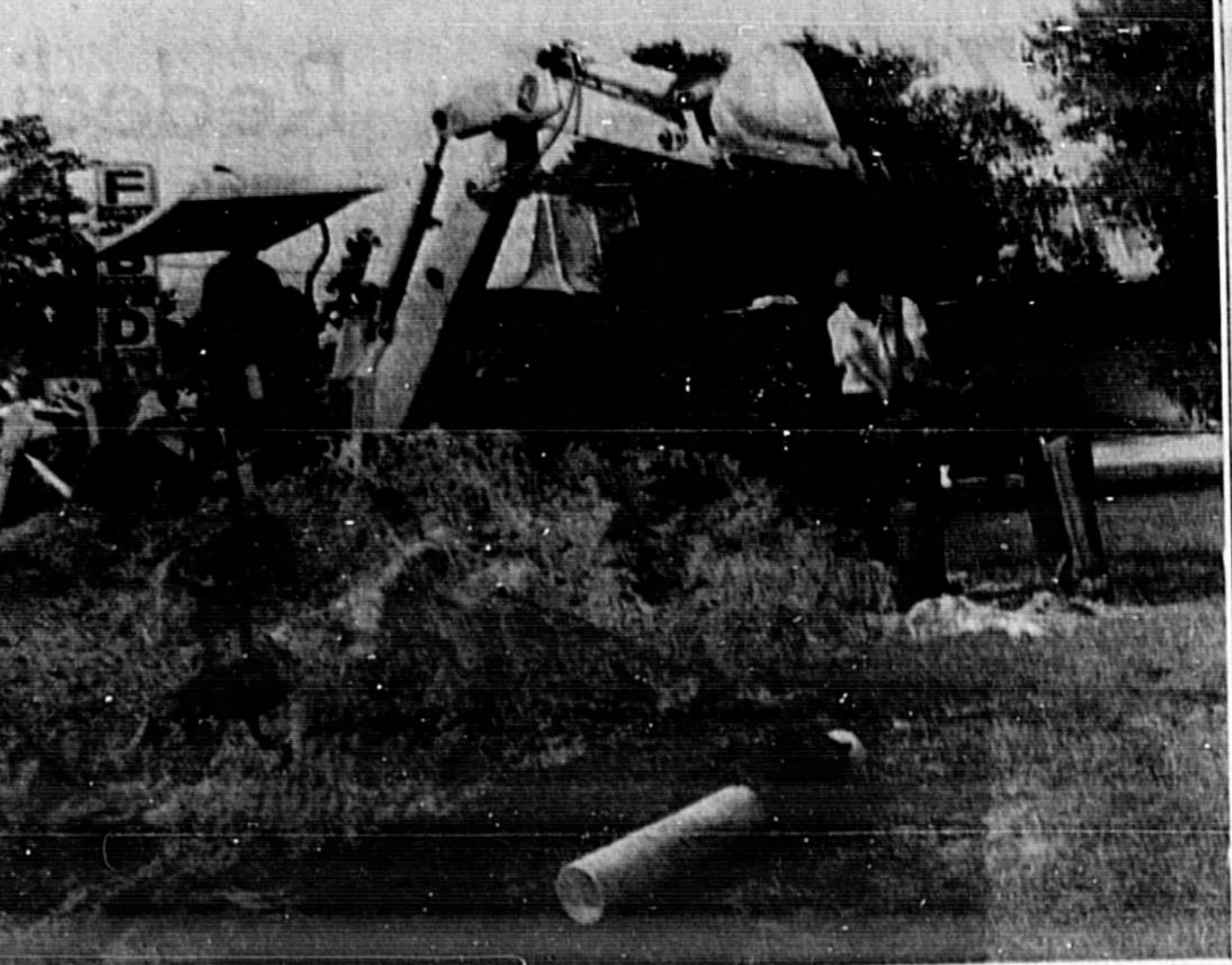
FIRST Bank of Deltona led the way in showing fire protection and fire prevention go hand in hand during Fire Prevention Week as they installed a fire hydrant in a strategic location to give additional protection for the bank and its neighbors. Charles Johnson, president of the bank and Don Williams (left) fire chief of the Deltona Volunteer Fire Department prepare to set the hydrant in position. (Dot Drew Photo)
