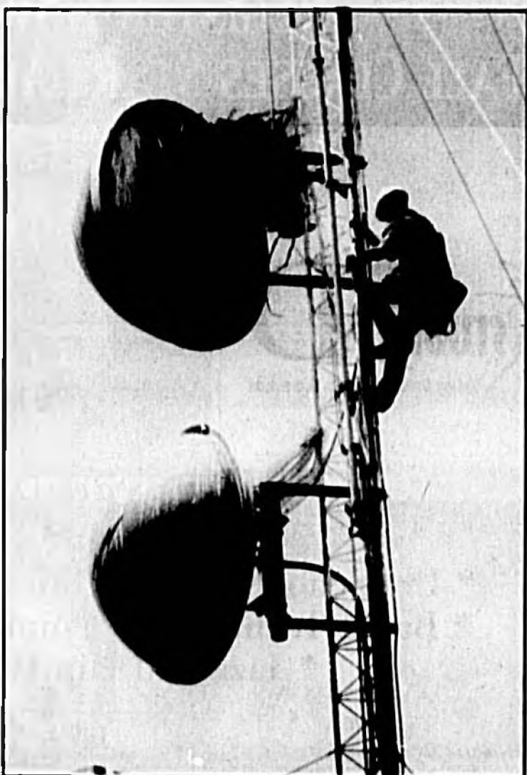
Steve Thomas, a tower hand for Tower Systems South Inc. of Winter Park, prepares to move a communications dish higher on the 100-foot towers atop the Seminole County Court House. Herald photo by Tommy Vincent
