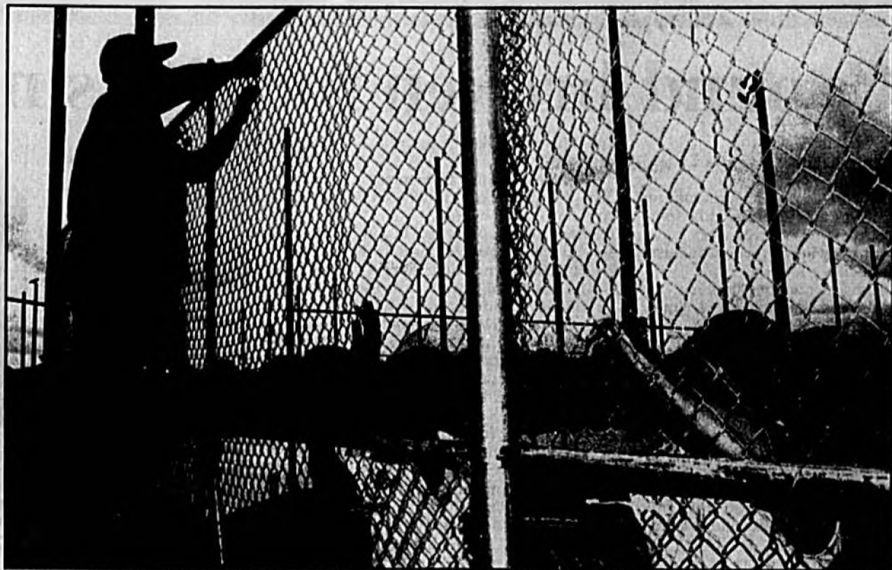
Work continues on the Chase Park Little League fields along Celery Avenue in Sanford. The city is in the process of building four separate ball fields. The work should be completed by March, which is the beginning of the Little League season. Installing a new fence around one of the fields are, from left, Randy Guay, job superintendent; Mark Tuoclarone, and Ron Hawkins. The men work for Federal Fence Company, DeBary.
