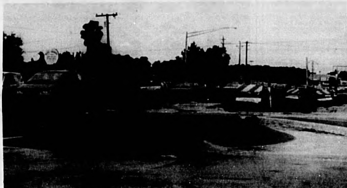
A volcano-like eruption of a water line on U.S. Hwy. 17-92 at Airport Boulevard tied up traffic Thursday.
