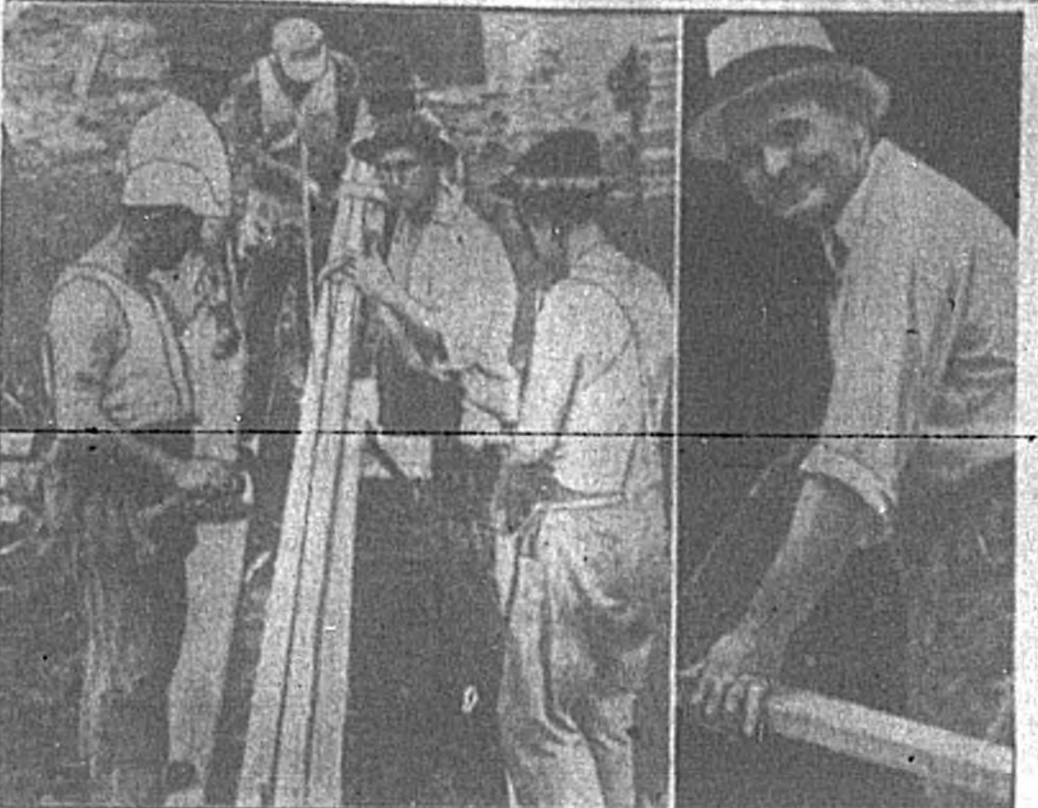
Rushing erection of Camp Franklin Roosevelt, near Ocala, Fla., carpenters are shown building the base for the $146,000,000 cross-Florida canal. On the right is Representative A. B. Folks of Marion county, who took a job as carpenter on the project and earns the same salary as he does as a member of the Florida legislature—$4 per day. (Associated Press Photo)
