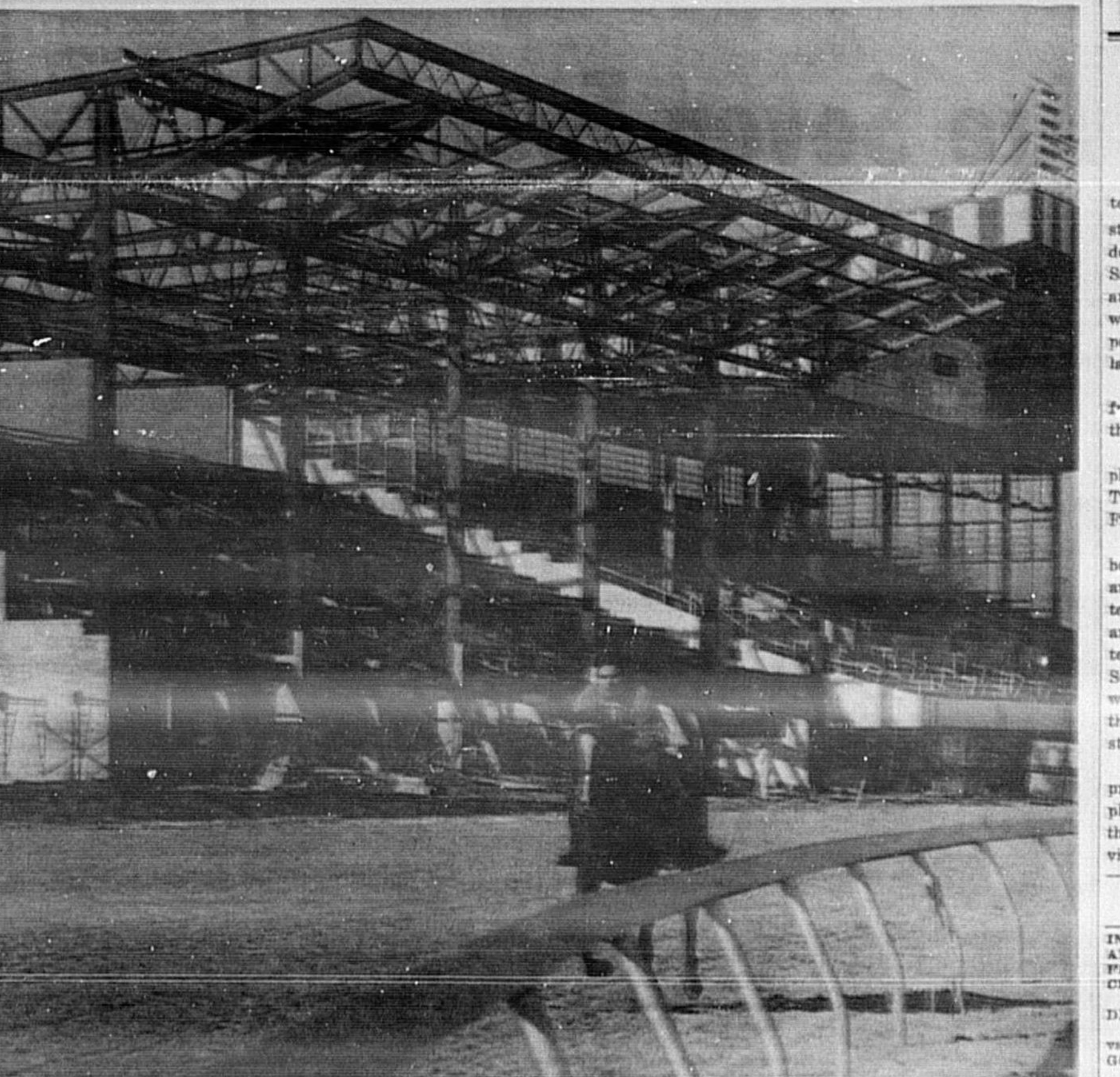
STEEL GOING UP — The $15 million clubhouse under construction at the Seminole Turf Club in nearby Casselberry forms a backbone for a thoroughbred working over the racing strip. Seminole will reopen April 20 for a 90-night thoroughbred meeting. New operators who acquired the plant last year are completely modernizing it at a cost of $2.5 million. The air-conditioned clubhouse will seat 800 diners at tables overlooking the stretch.
