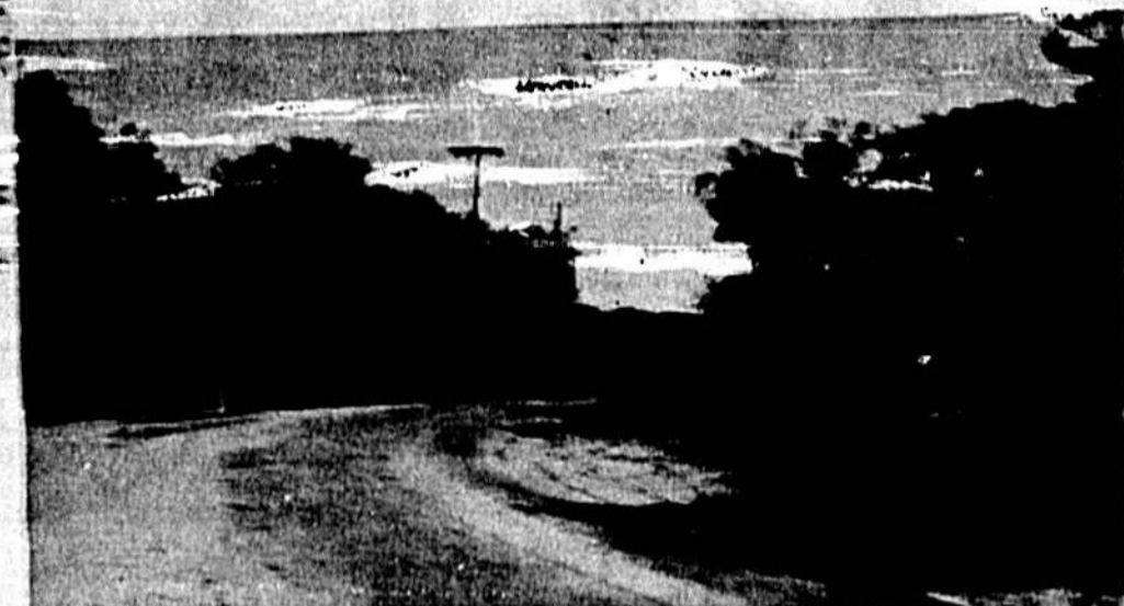
LARGE TREES have been uprooted in the path of new SR 426 from Oviedo to Goldenrod. The roadway will be straightened to eliminate sharp curves. (Herald Photo)
