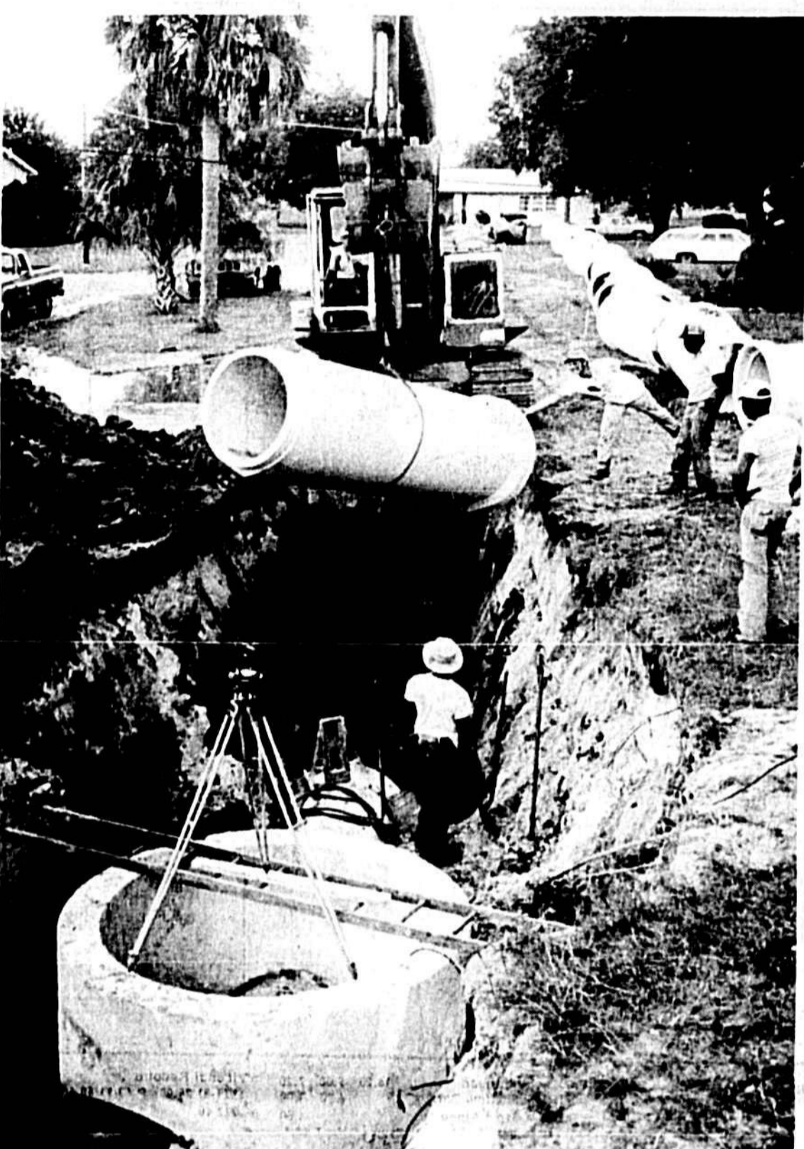
Workmen install a pipe near the Good Samaritan Home on Ninth Street in Sanford. The pipe project is part of a $153,000 community development project designed to help eliminate flooding in the Goldsboro basin.
