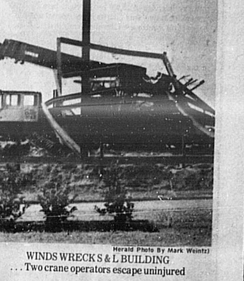
WINDS WRECK S & L BUILDING Two crane operators escape uninjured
