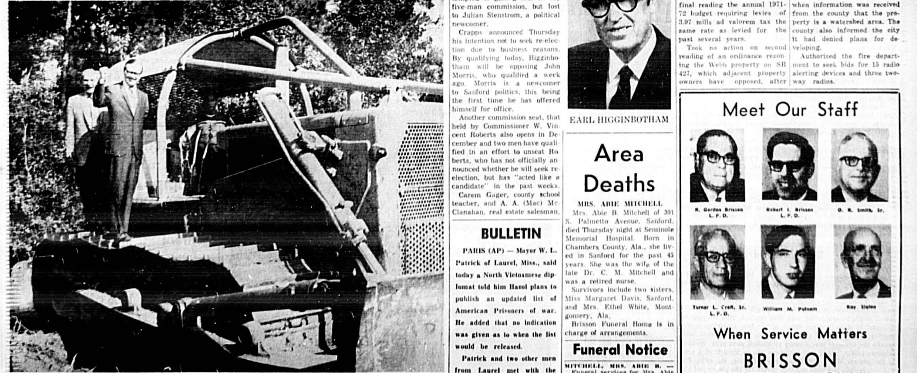
AT LONG LAST — So cheer two Greater Sanford Chamber of Commerce officers as this giant bulldozer this morning started moving dirt in the construction of a new State Road 46 between Interstate 4 and the Wekiva River. Douglas Stenstrom (front) and John Krider are among the many civic leaders who pushed for more than a decade seeking the new highway. The $860,000 project is scheduled for completion in about nine months. (Bill Vincent Photo)
