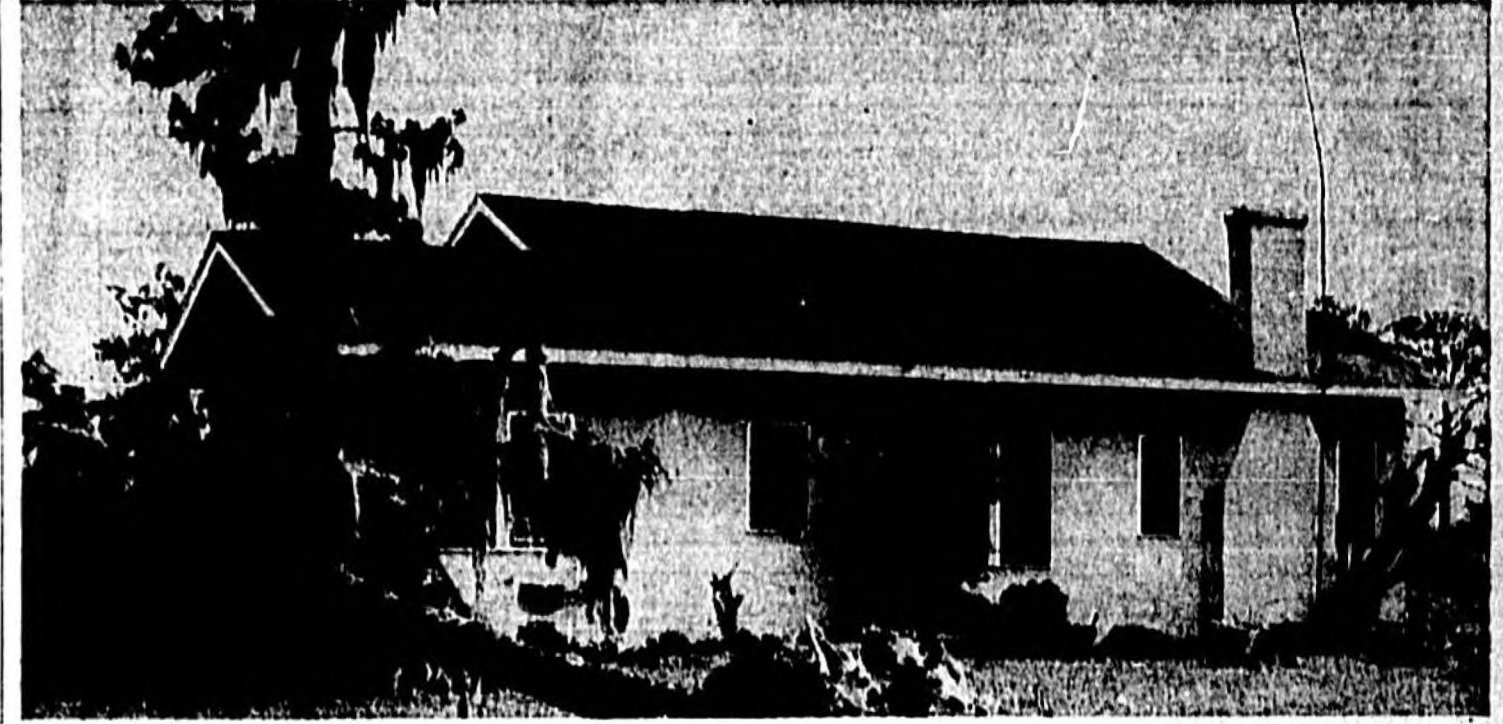
A TORNAIDO-LIKE STORM whipped through South Sanford yesterday afternoon blowing over trees and ripping roofs. Above photo shows a tree blown over on the home of Clarence Wynn, 2006 Grandview Ave. Notice the bent TV antenna. The damaged area covered a four or five block area east and west across the city. (Photo by Bergstrom)
