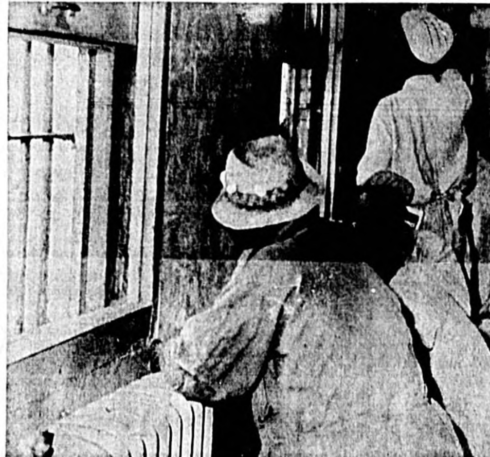
WORK STARTED THIS morning on renovating the old county jail into a first class city police station. The first step in the $12,000 program is the scraping of old paint on the top floor. The job is expected to be completed in two months. (Herald Photo)
