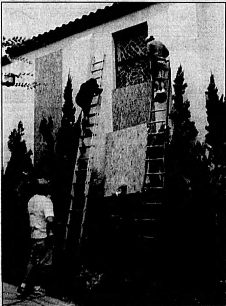
By installing anchors and pre-drilled holes during good weather, maintenance crews at All Souls Catholic Church can quickly install pre-cut sheets of plywood to protect the church's stained glass windows..
