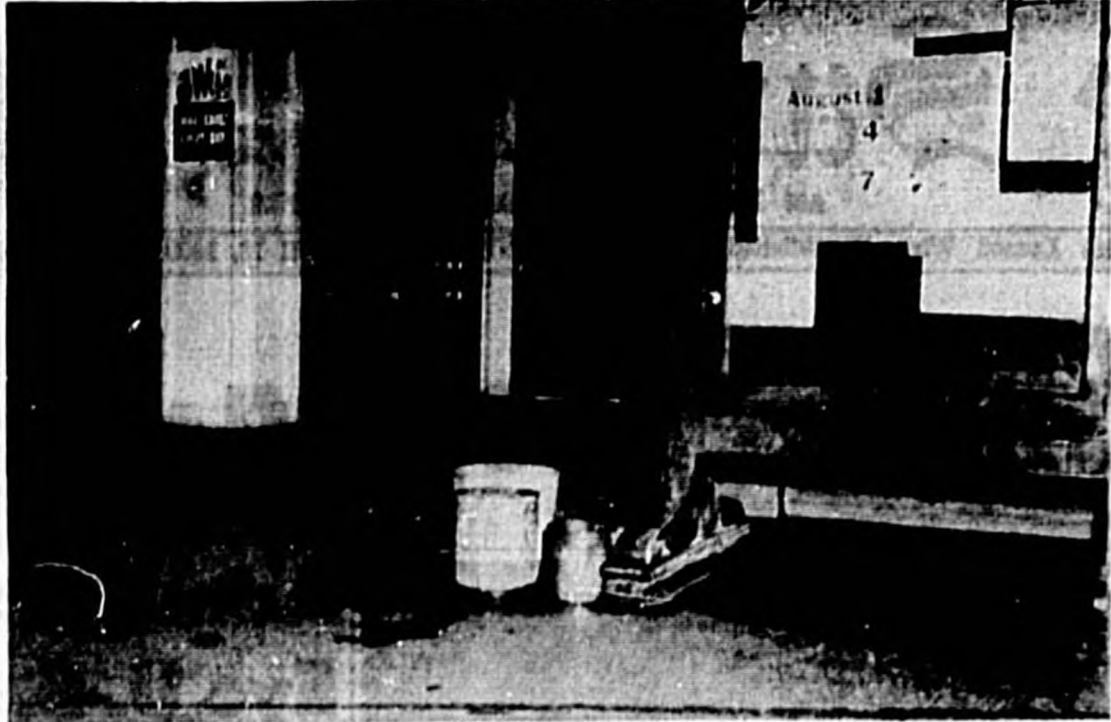
RAIN CATCHERS —This is a typical scene in from small holes in the ceiling of the Post Office. Altogether, there are five buckets catching the rain leaking in from small holes in the ceiling of the Post Office. (Herald Staff Photo)
