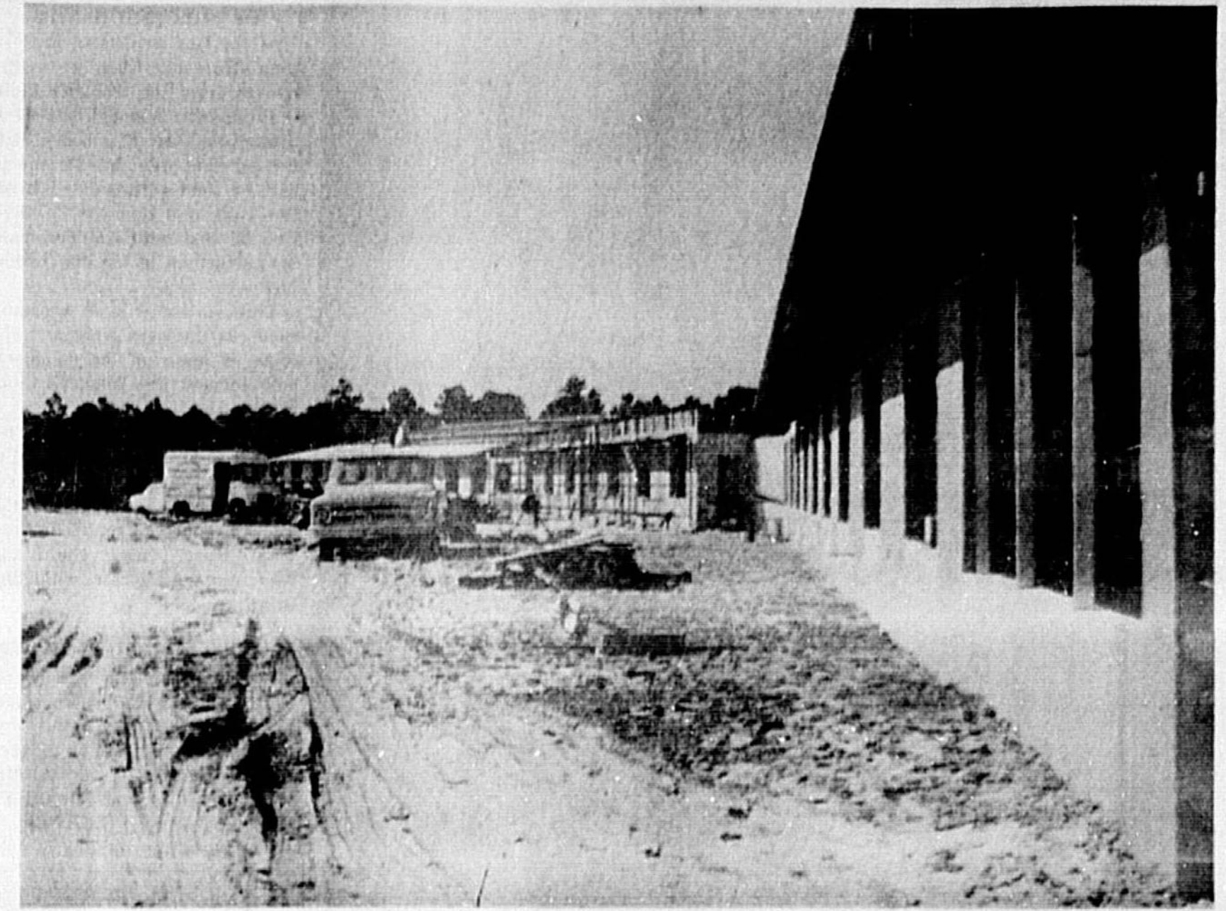
WORK IS coming along on the Florida Living nursing center at Forest City. This is to be an 108-bed nursing home, at a cost of $1,072,000. It is a project of the Seventh-day Adventists and is hoped to be completed by early 1970. Van McGlawn will be the director of the center. (Maryann Miles Photo)
