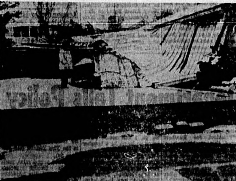
MRS. MARVIN PUTNAM surveys the damage after a heavy snowfall collapsed the roof of her patio at La Crescenta, Calif. It was the first snow to fall in the area in five years and the weatherman said more is on the way. (NEA Telephoto)
