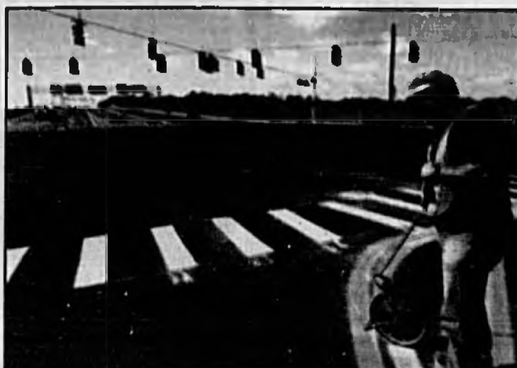
Robert Weinbender of the Department of Transportation measures striping at the new SR 46A interchange, which opens today. The interchange will provide an additional Sanford exit off of Interstate 4. A ceremony will be held at a later date.
