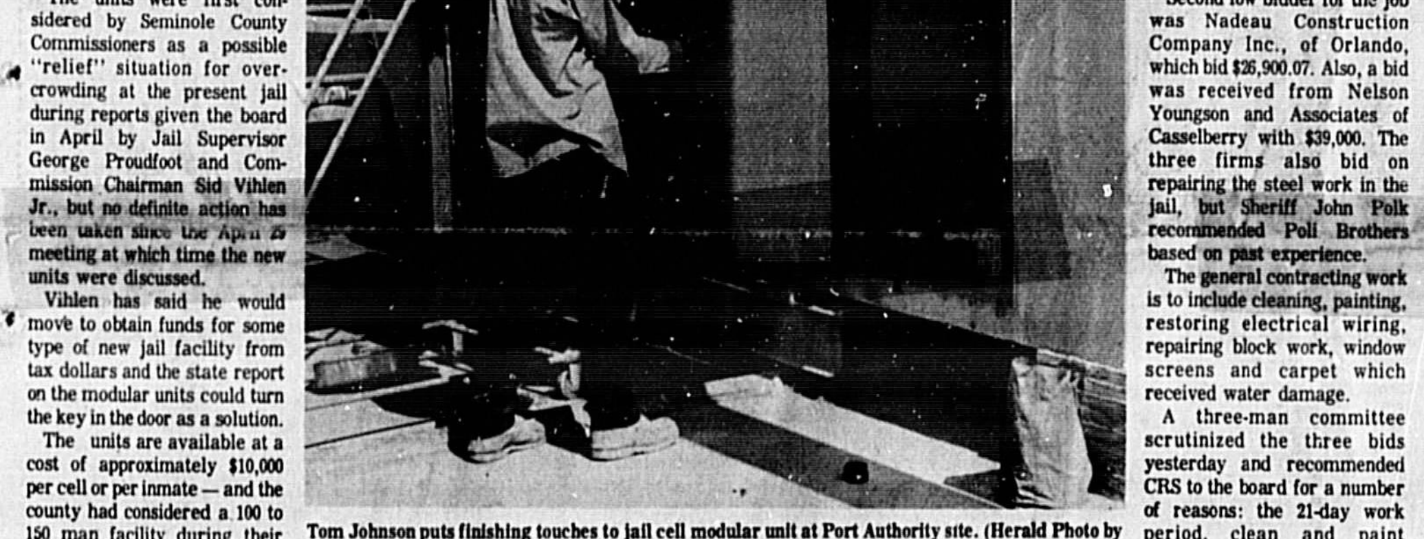
Tom Johnson puts finishing touches to jail cell modular unit at Port Authority site.
