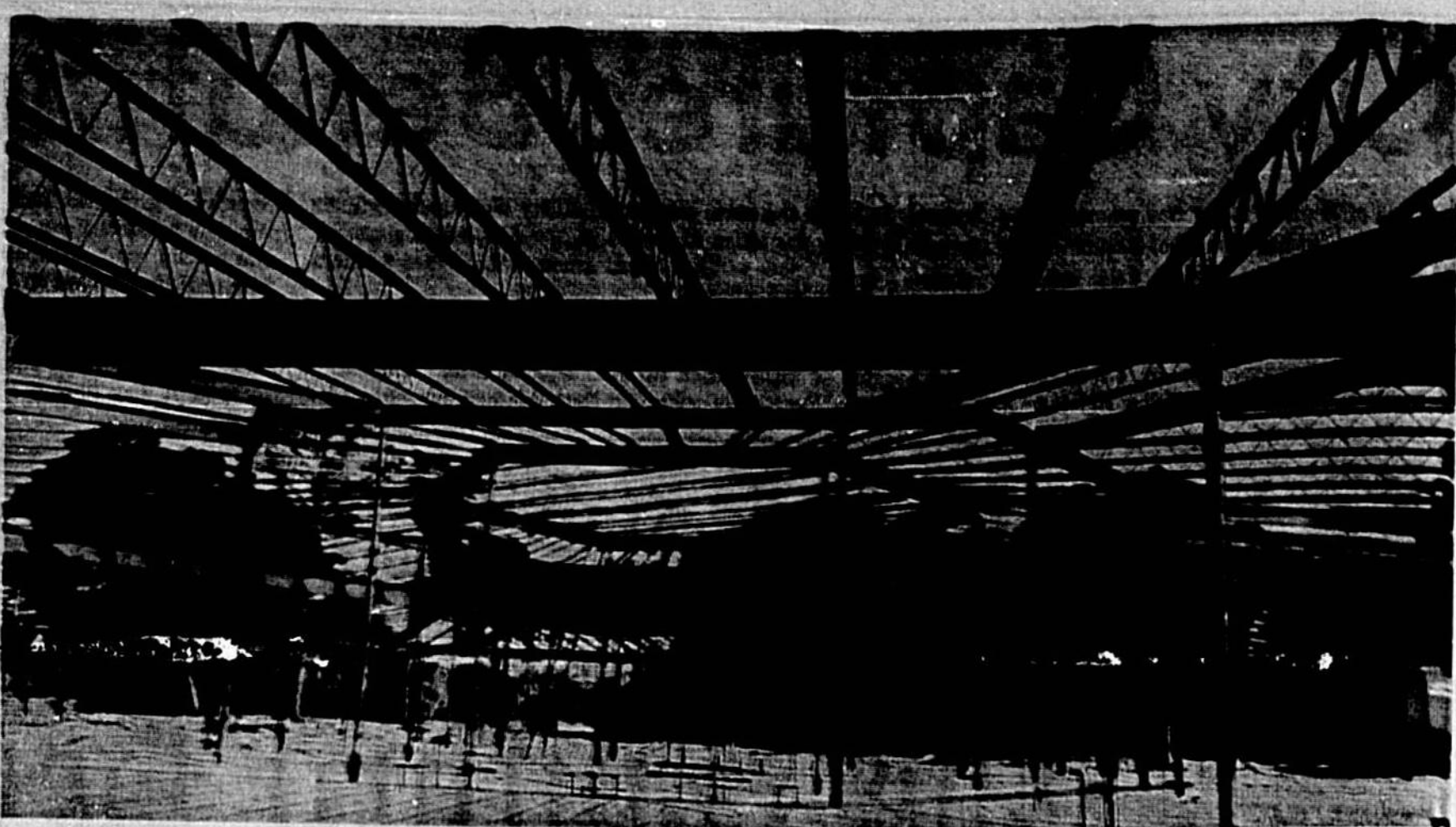
SPIDERWEB effect is created in this Bill Vincent Jr. photo by the steel framework of a new Sanford Junior High School building. This hexagon-shaped building will be occupied by classrooms, laboratories and temporary administrative offices and will be ready for occupancy next September. This plant will house 700 students, or 40 per cent of the total school population in the ultimate facility. (Herald Photo)
