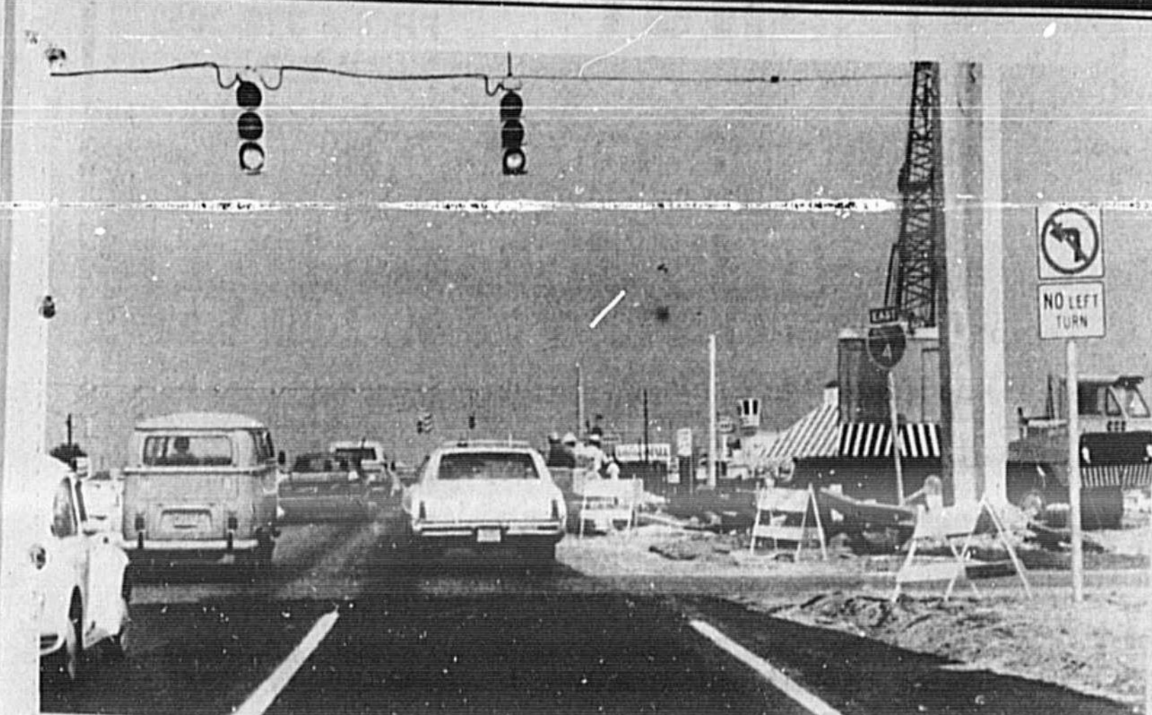
ALTAMONTE'S TRAFFIC JAMMED Revamping of the SR 436 bridge over Interstate 4 in Altamonte Springs from four lanes to seven much traveled intersection. Completion of the job, tied in with other area road improvements, however, is expected to take 12 more months. Rather than two lanes in either direction, the revamped bridge will also have two left turn Westbound lanes onto I-4 and one left turn eastbound lane to I-4. A traffic count by the state Department of Transportation prior to the opening of the Altamonte Mall last summer at the I-4-SR 436 spot showed 35,000 vehicles per day going through the intersection.
