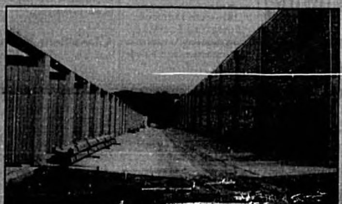
The mini warehouse complex now under construction on SR 46 in Sanford will include climate control storage units. Completion of Phase I is scheduled for October.
