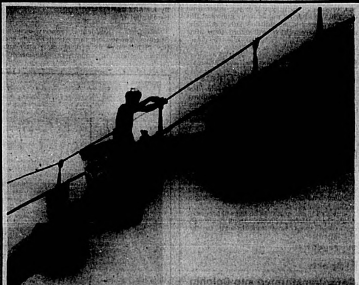
New sign Airport Boulevard became easier to find Tuesday with the help of Bob Loyer, Control Specialists Co., of Orlando had replaced the traffic lights at the intersection of U.S. 17-92 and Airport Boulevard, and a new directional sign seemed to top the job off.
