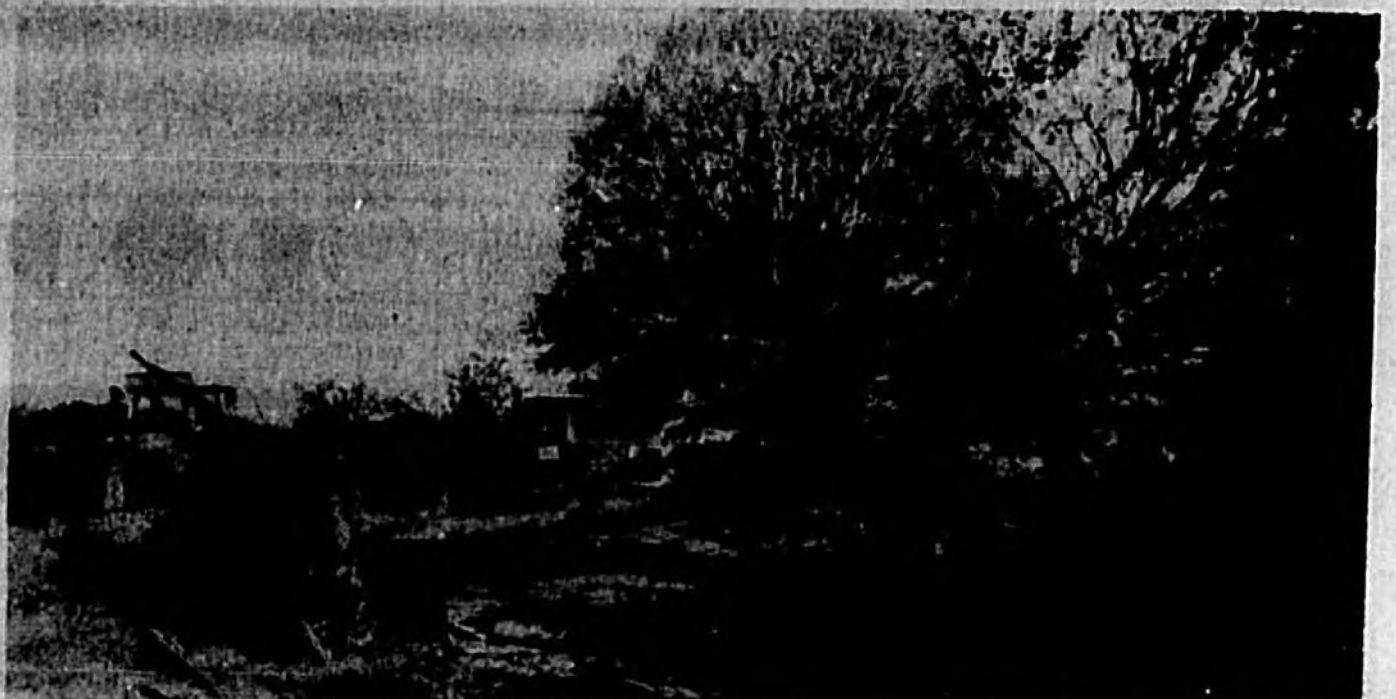
Workers prepare to haul away tree cut down to make way for an airport fence.
