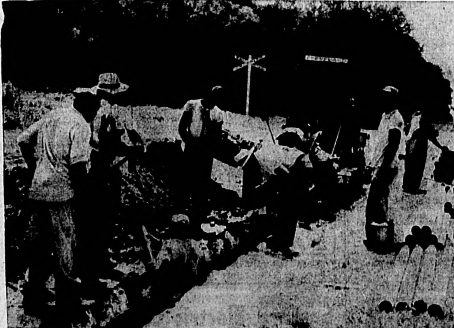
UNDERGROUND SUBWAY IS being installed for cables to re-center the telephone exchange to the new telephone building and to provide additional service to many customers after conversion to dial next March 17. Approximately 40,000 feet of nine duct subway extending from Ninth St. and Laurel Ave. East to Palmetto Ave. and South on Elm Ave. to 10th St. is being installed with eight manholes at a cost of $63,000. This is one of many projects to be completed during the next six months so that the best possible telephone service can be given to Sanford subscribers. (Photo by Jameson)
