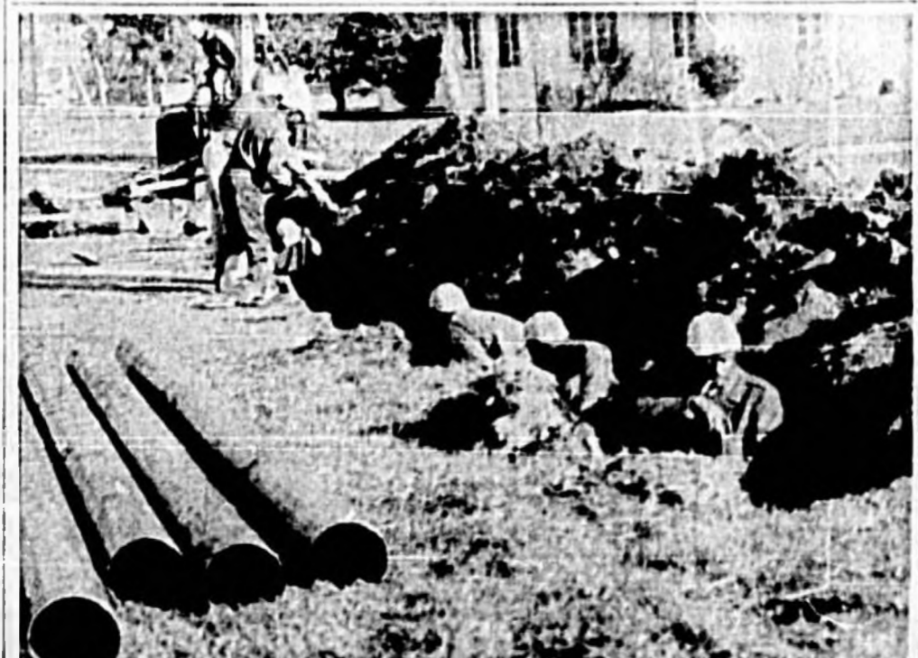
CITY CREWS TODAY started the first step in the construction of the jet fuel pipeline to the Sanford Naval Air Station by putting down casing at the intersection of Mellonville Ave and Randolph St. The Sanford Pipeline Co. will open bids on the two mile stretch later in the month with construction to start soon afterwards. (Herald Photo)
