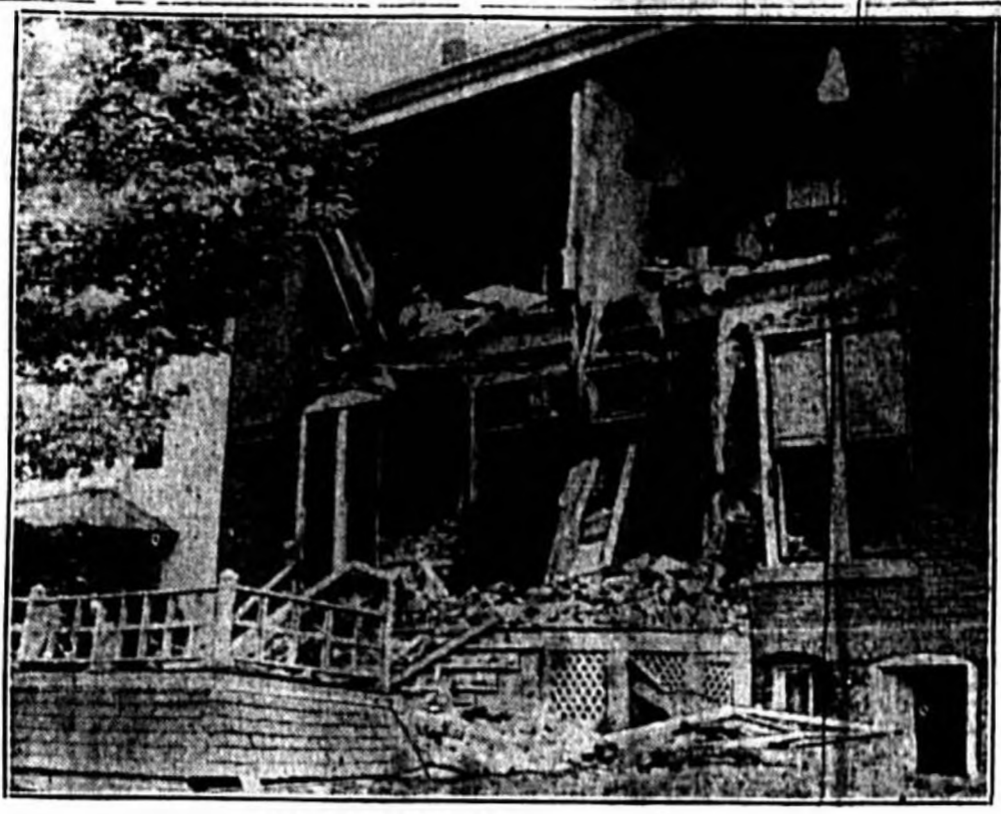
When an earthquake rocked Helena, Mont., killing two persons and doing damage of $1,000,000, the home of Edward Rittig was shaken to pieces, as this picture shows, but a member of the family sleeping in the upper front bedroom escaped uninjured. (Associated Press Photo)
