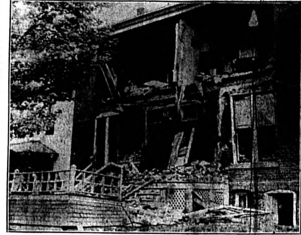
When an earthquake rocked Helena, Mont., killing two persons and doing damage of $1,000,000, the home of Edward Reing was shaken to pieces, as this picture shows, but a member of the family sleeping in the upper front bedroom escaped unharmed. (Associated Press Photo)
