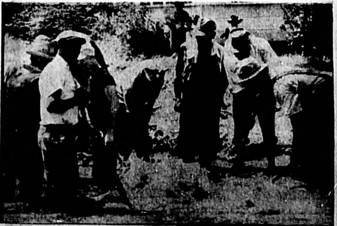
CITY CREWS PUT an eight-inch water main back into operation at First St. and French Ave. Saturday morning. Workmen are removing dirt and sand from around the pipe preparatory to the repair. (Staff Photo)
