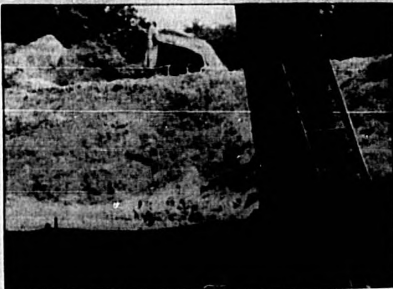
The view in Loch Arbor used to be of trees, but The Mayfair Club project has leveled them. The area has been built up so new homes will sit above the old neighborhood causing existing residents to fear problems with flooding.
