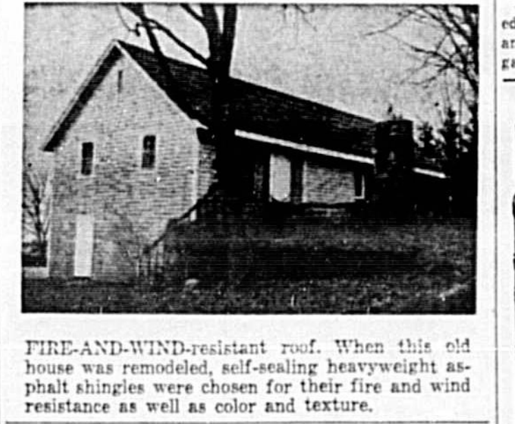
FIRE-AND-WIND-resistant roof. When this old house was remodeled, self-sealing heavyweight asphalt shingles were chosen for their fire and wind resistance as well as color and texture.
