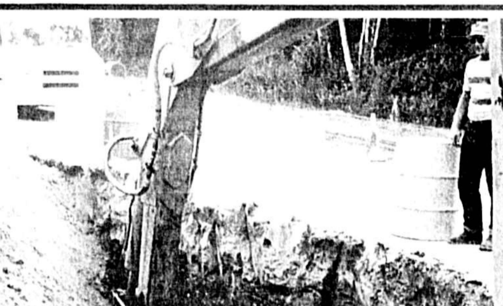
Base Paving & Construction Co. crews remove muck in Winter Park Drive project in Casselberry.
