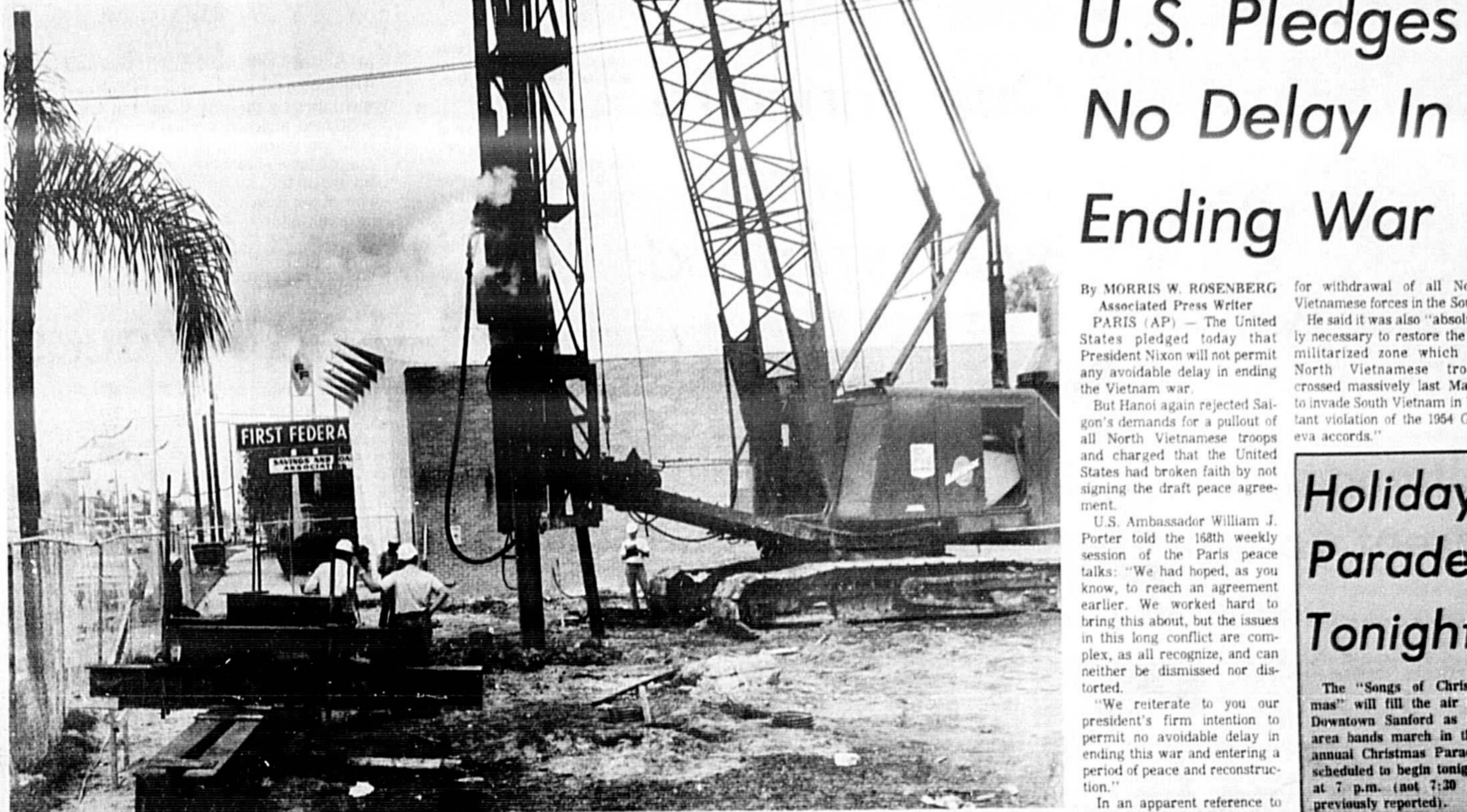
HOW FIRM A FOUNDATION Pilings—over 100 of them—are being driven to provide a solid foundation for the four-story addition to First Federal Savings and Loan Association's First Street facilities. This latest step in improving and modernizing Downtown Sanford will cost over a $1 million. (Staff Photo)
