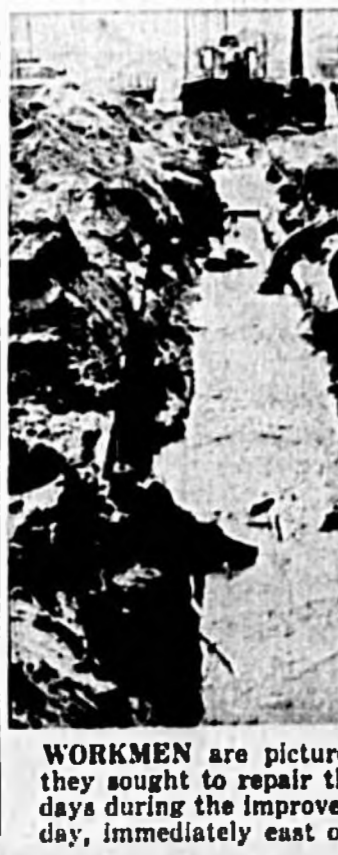
WORKMEN are pictured knee-deep in water Wednesday afternoon as they sought to repair the third rupture of the city water pipeline in 10 days during the improvement program of 25th Street. The break Wednesday, immediately east of Park Avenue, also disrupted telephone service.
