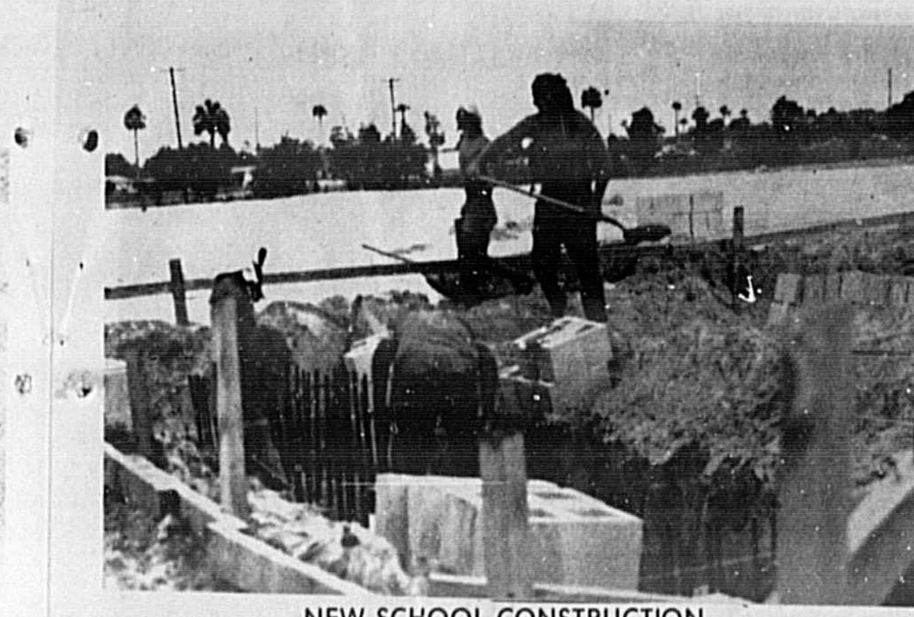
NEW SCHOOL CONSTRUCTION WORKMEN ARE shown preparing foundation for new $950,000 Winter Springs Elementary School on SR 44. Until the facility is completed in January the student body and faculty will attend double sessions at Red Bug Elementary School. David Sawyer will be principal of the new kindergarten through fifth grade school, designed to accommodate 600 students.
