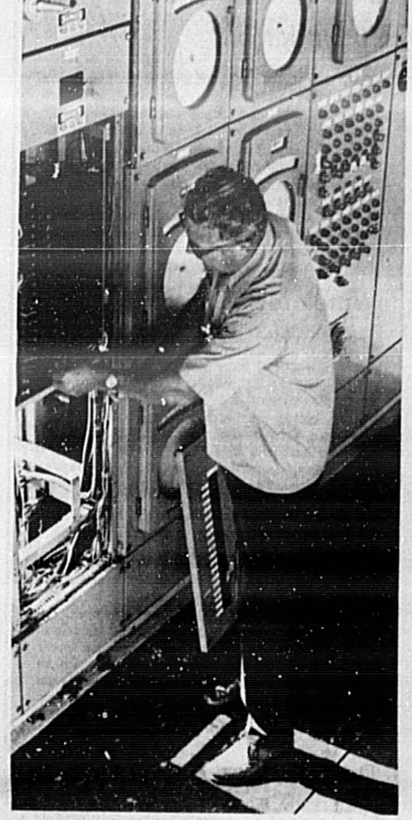
RICHARD CHECKS POWER PANEL ... Plant back in operation
