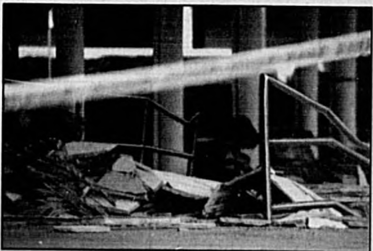
Rubble remains piled up from the breezeway ceiling leading to the entrance of St. Mary Magdalen Catholic Church in Altamonte Springs. Twenty-three parishioners were injured Sunday when the ceiling collapsed shortly before the scheduled noon Mass. See Russ White's column on Page 3A for more on this story.
