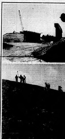
None Too Soon These concrete pilings (above) will be driven into the ground as the foundations for the railroad overpass on State Road near the currently under construction just west of Sanford and at the Amtrak and auto-train terminals. A crew is working to lay out on one of the overpass' two embankments (all left) to retain the soil. Completion for the overpass is tentatively set for January 1964. The work is being done by RKG Inc. of Burlington, N.C., under the direction of the state Department of Transport. The cost of the improvements is $2.46 million, paid in part by a federal grant. The completion of the improvement will be none too soon.
