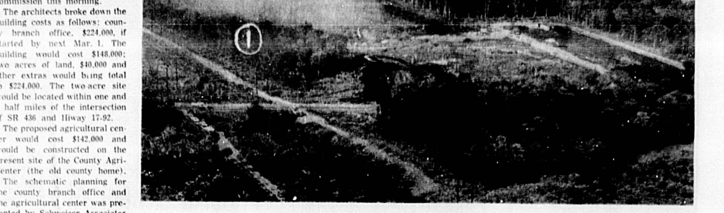
SANFORD PORT site from the air is pictured. Cleared area (center) will be occupied by the wharf and warehouse. Area covered by trees and smoke (No. 1) will be the barge basin, itself. Sixty-foot concrete pilings have been driven to test
