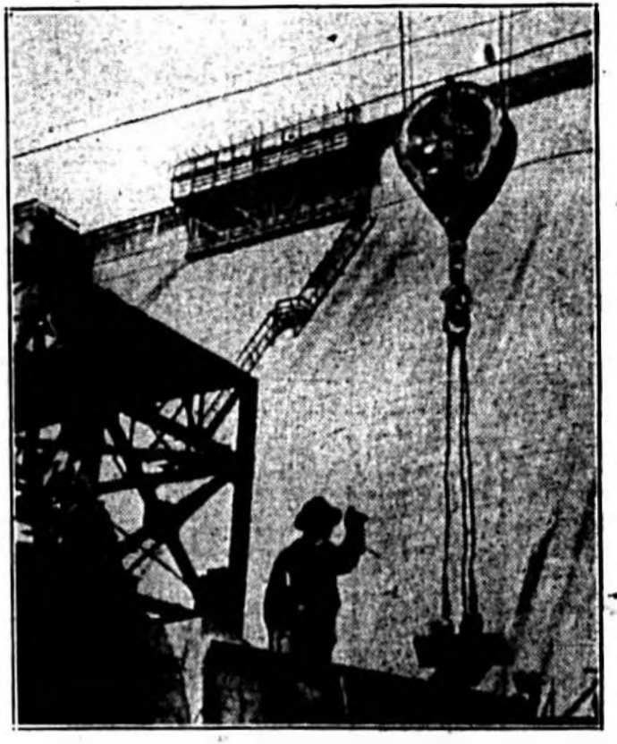
These workmen and machines at Norris dam near Knoxville, Tenn., will continue at full speed, now that the United States Supreme Court has ruled in favor of the Tennessee Valley Authority in litigation disputing the federal government's right to sell surplus power manufactured at TVA dams. The decision was a major victory for the New Deal. (Associated Press Photo)
