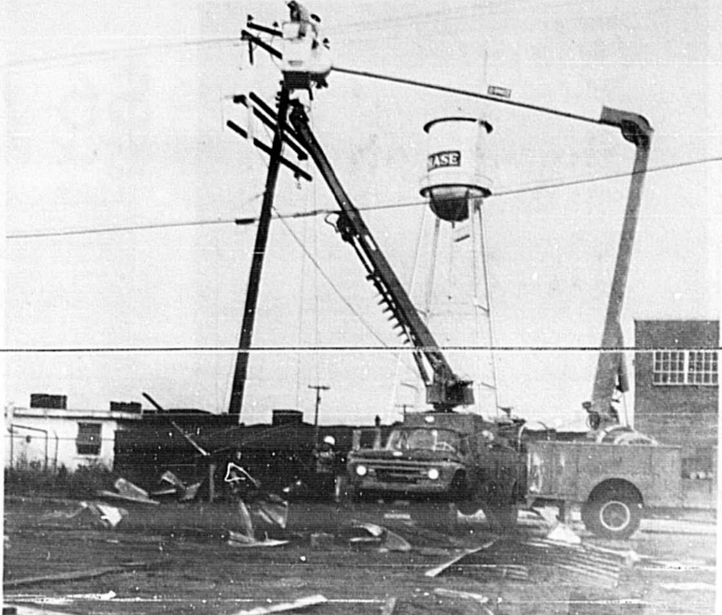
FLORIDA POWER and Light workers untangle a mass of lines after a twister hit a building on Beardall Avenue, east of Sanford, yesterday afternoon. One pole was snapped and several wires blown or tangled by the high-winds. The building was a warehouse owned by Chase and Company and was totally destroyed. Lee Moore, vice-president of the company, said items in the building included agricultural chemicals, seeds and cabbage bags. (Gary Taylor Photo)
