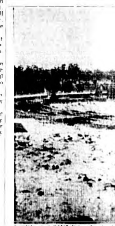
WORK CONTINUES—In the logging afternoon, work continues on Sanford's expanding water and sewage system. The Hobson Construction Co. is shown laying water pipe by the Memorial Stadium on Melbourne Ave. to what eventually will be the new water tank. Foundations for the tanks of structure can be seen in the foreground. (Staff Photo)
