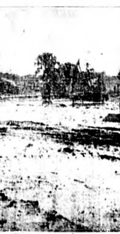
WORK CONTINUES—In the logging afternoon, work continues on Sanford's expanding water and sewage system. The Hobson Construction Co. is shown laying water pipe by the Memorial Stadium on Melbourne Ave. to what eventually will be the new water tank. Foundations for the tanks of structure can be seen in the foreground. (Staff Photo)
