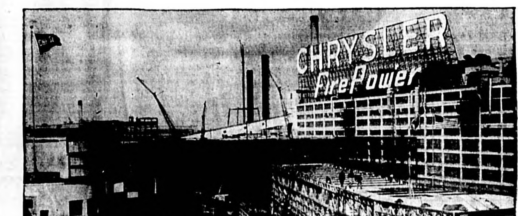
UP GOES CHRYSLER'S PRODUCTION MORE THAN 40% Here you see construction work proceeding on the new Chrysler production facilities which will add 847,000 square feet of floor space... including a 14-mile long continuous conveyor system, located in the building.
