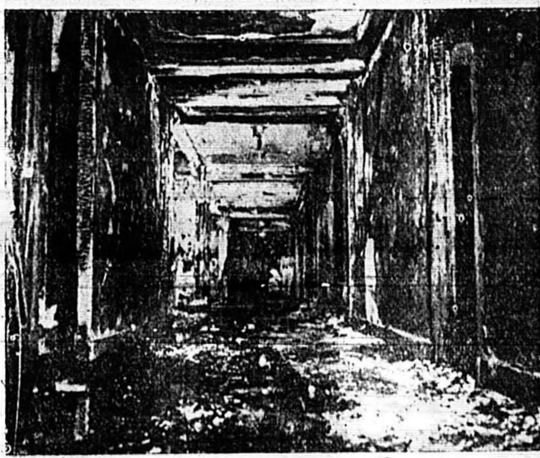
HERE IS A GENERAL VIEW OF THE GUTTED HALLWAY OF THE 12-story La Salle Hotel in Chicago. At least 54 persons died in the hotel fire, worst in Chicago's history. Approximately 200 persons, including 30 firemen, were overcome by smoke or suffered burns and injuries.
