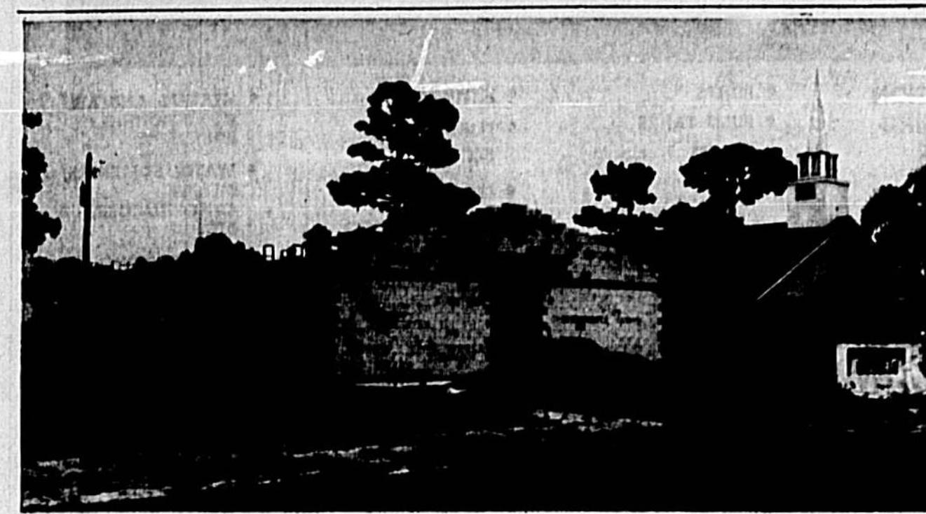
NEW SANCTUARY for First Baptist Church of Lake Mary, one of Seminole County's oldest communities, is shown under construction. Completed in time for the congregation's October revival, the new building is air conditioned throughout and has a 450 person seating capacity. People from the former sanctuary, seen at right in photo, has been removed and this building has been converted into classrooms. (Herald Photo)
