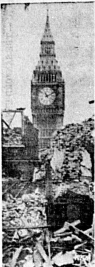
REMINISCENT of the Battle of Britain during World War II, Big Ben rises from the ruins of a demolished building. Actually, however, this structure near London's famous clock is being torn down in a modernization program.
