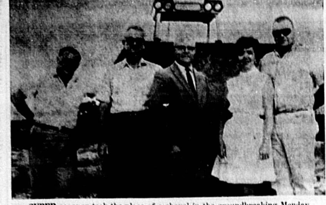
SUPER scooper took the place of a shovel in the groundbreaking Monday for the new Uniroyal Auto and Home Center on I-92, Casselberry. Mayor Curtis Blow (center) participated together with Ted Chapman, equipment operator, George Fisher, Fisher Construction Company; Gerald D. Blyeu, project co-ordinator for Tavaglione Construction Company, and Mrs. Blyeu.
