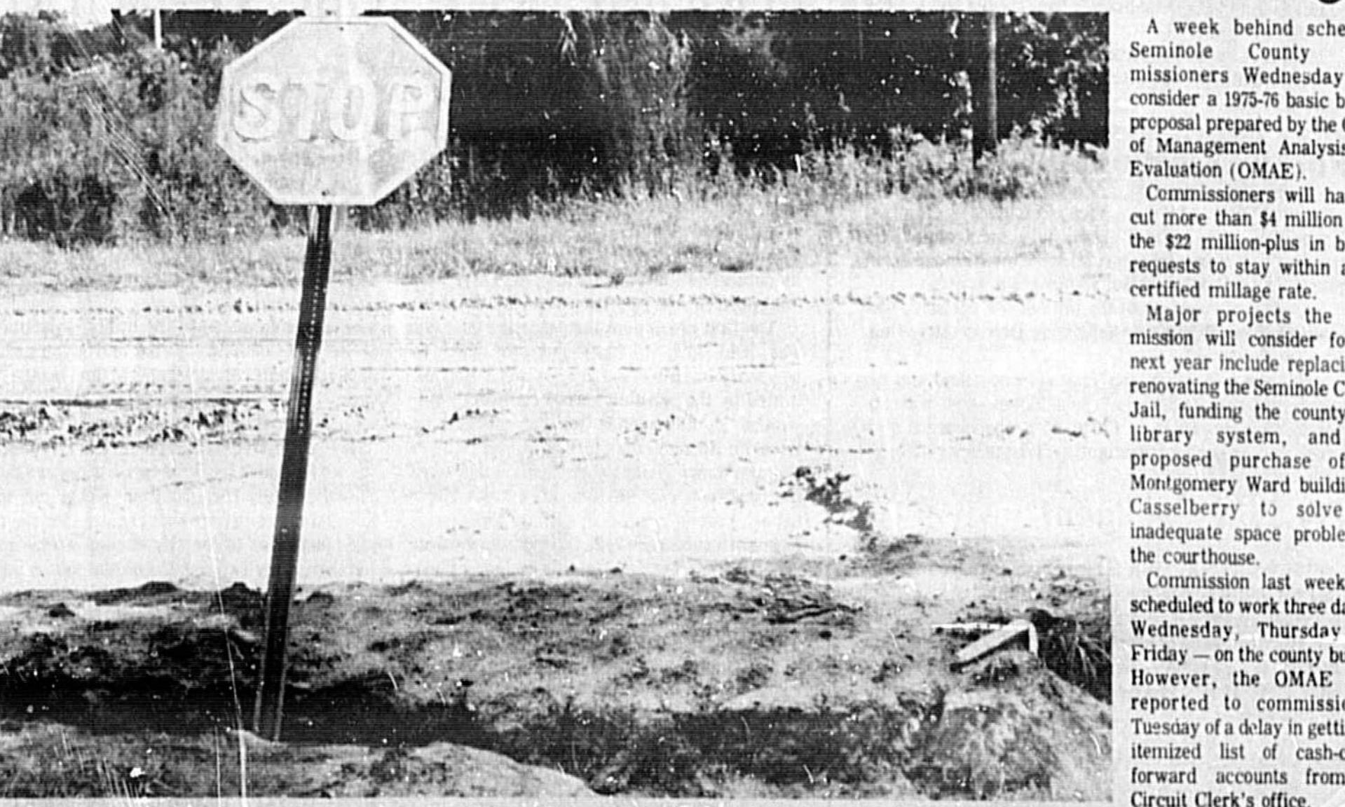
ANOTHER CAVE-IN Numerous cave-ins and sinkholes have been created throughout the city of Sanford in recent weeks, due to unusually heavy rains and thunderstorms. This one happened at the corner of 24th Street and Chase Avenue and caused the stop sign to go topsy-turvy. City maintenance crews are working as rapidly as possible to fill in the washed away earth, but more rains could cause more problems. The weekend weather forecast is calling for 40 per cent chance of afternoon and evening thundershowers. (Herald Photo by Bill Vincent)
