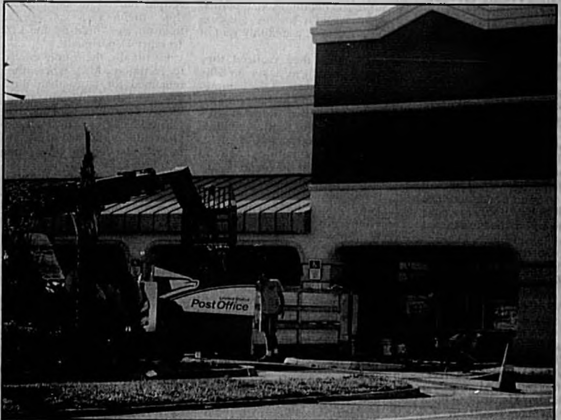
Workers install signs at the new Sanford post office, located at the corner of 1st Street and Sanford Avenue. Crews are finishing up work at the site, and postal officials anticipate the facility will open within the next week.
