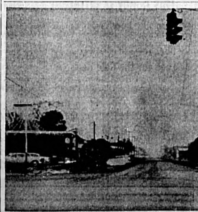
TAKING SHAPE is the four-lane section of First St. which is being widened from French Ave. to the intersection of Interstate 4. The picture shows the width of the $600,000 project which will give Sanford adequate access to the new expressway when it is completed. (Herald Photo)
