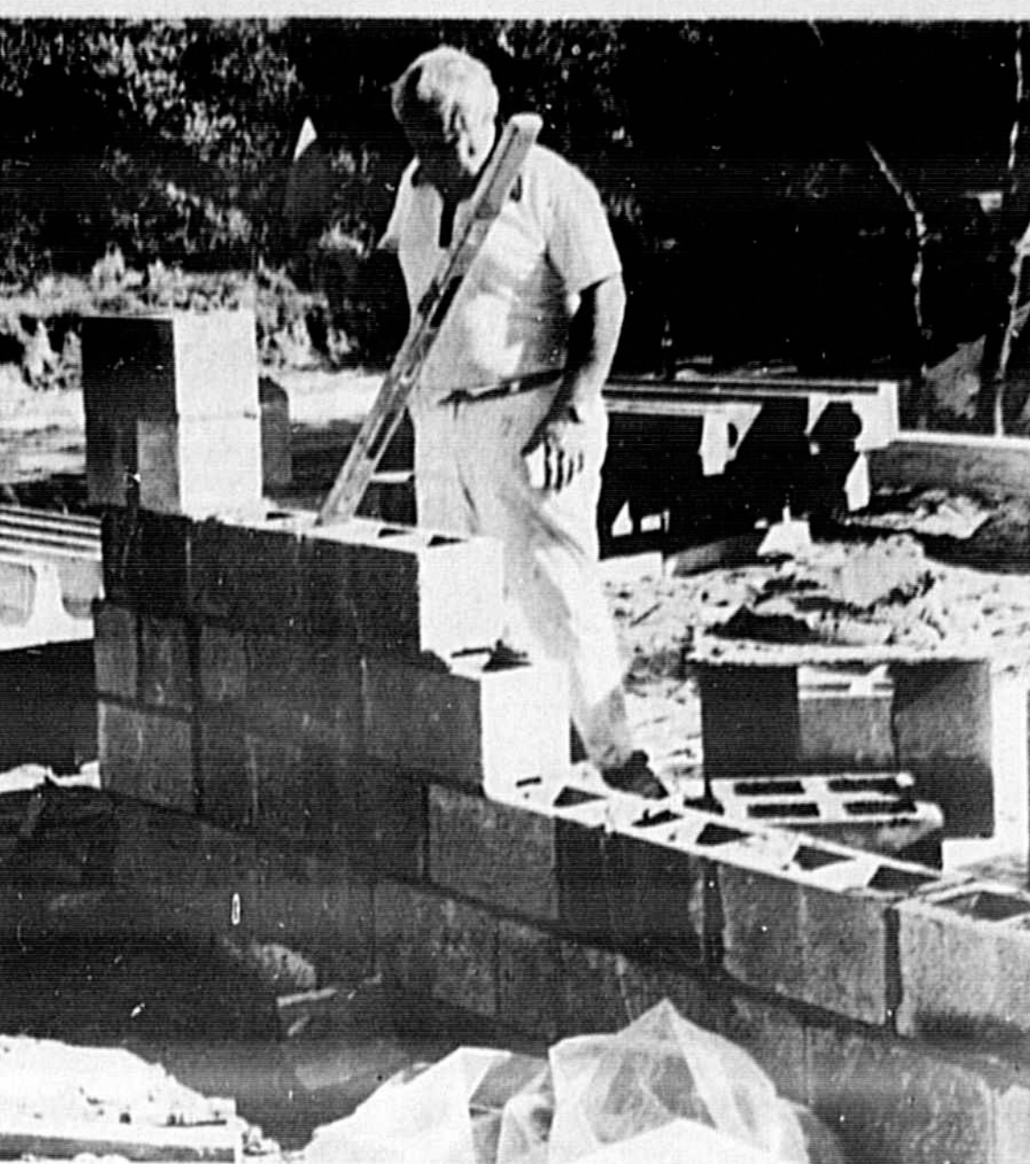
IF YOU DECIDE to build on that extra room yourself always be sure to have a good level handy when laying blocks. Now is the time for "Clean up - Paint up - Fix up."
